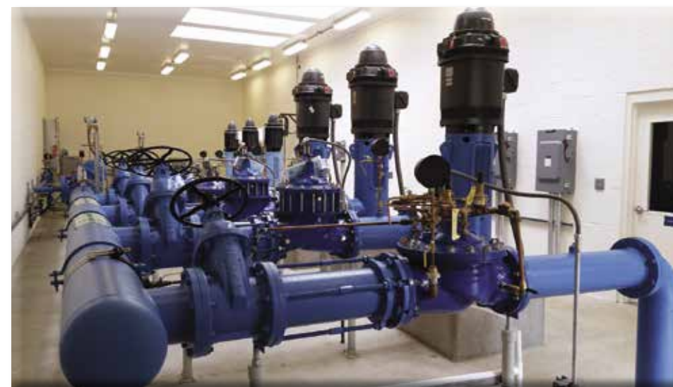
NESSWD Crest Treatment Plant that effectively filters detectable arsenic from our groundwater system. This facility is an additional method we use to ensure your water is the purest available.
